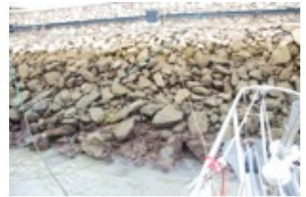
The wall off the bow - about 10 feet of tide which must be accounted for in the mooring lines
